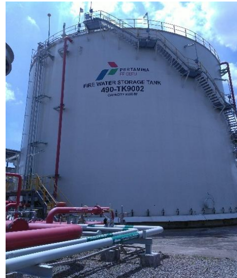
Gambar 5. Fire Water Tank
